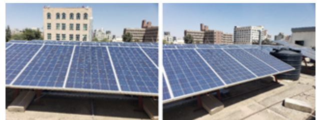
Figure 2. A section of the (P-Si) PV modules that are installed on the roof of the Yemen Standardization, Metrology and Quality Control Organization (YSMO) in Sana'a – Yemen.
